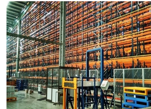
Automated Storage and Retrieval System
